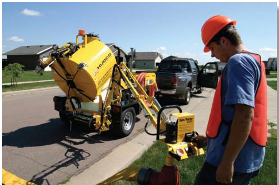
Exercise valves and hydrants quickly.
